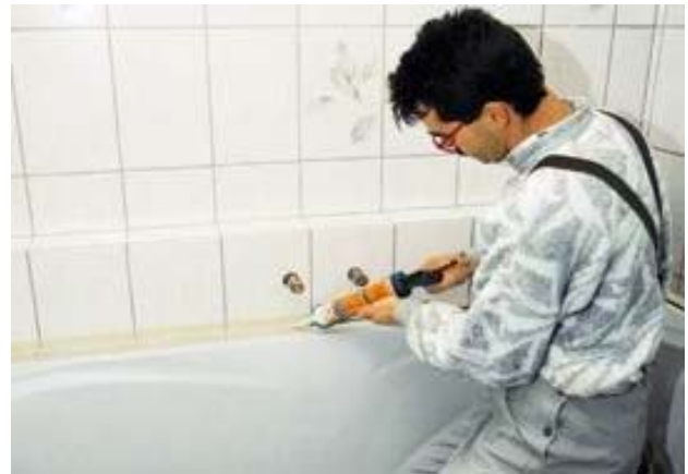
Elastic sealing of joints with PCI Silcoferm VE; colour shades match the grout.
